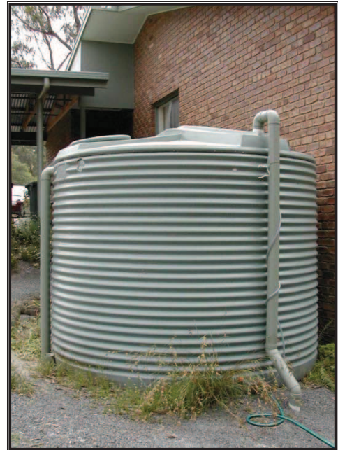
PLATE 6.6 – TYPICAL RAINWATER TANK
